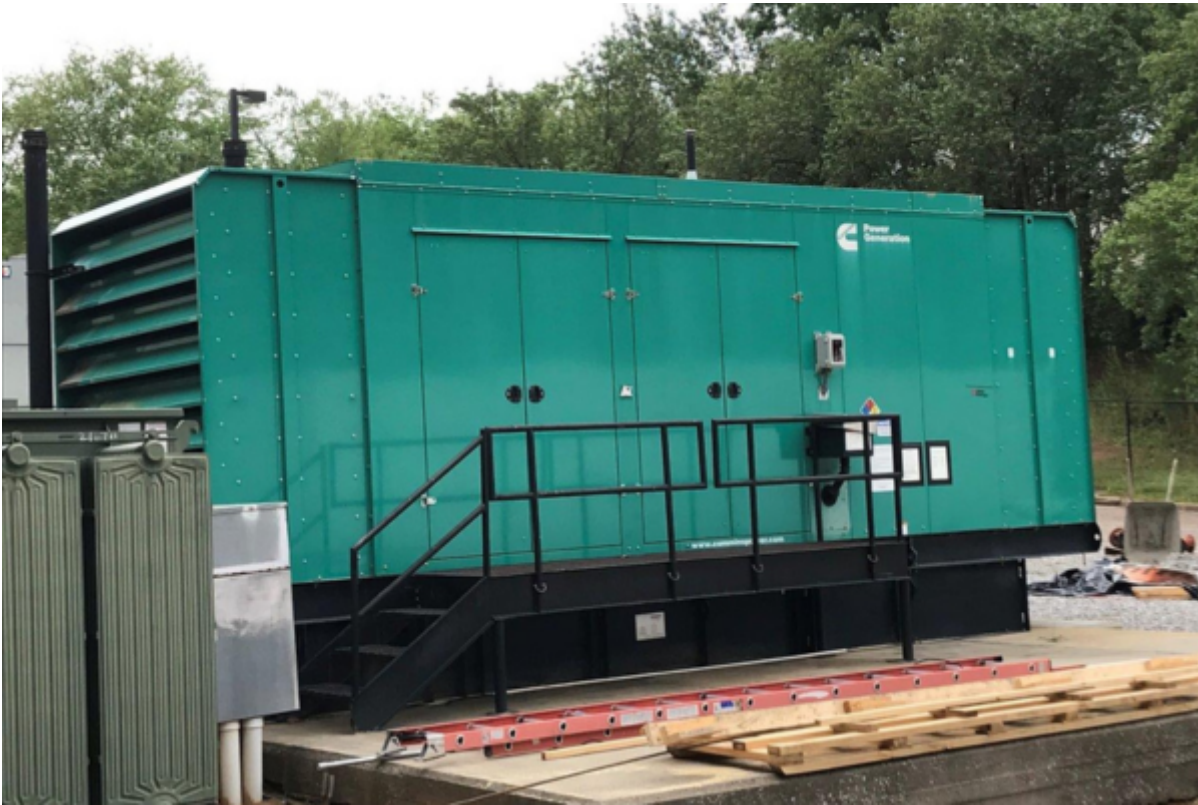
Industrial Power Generators
