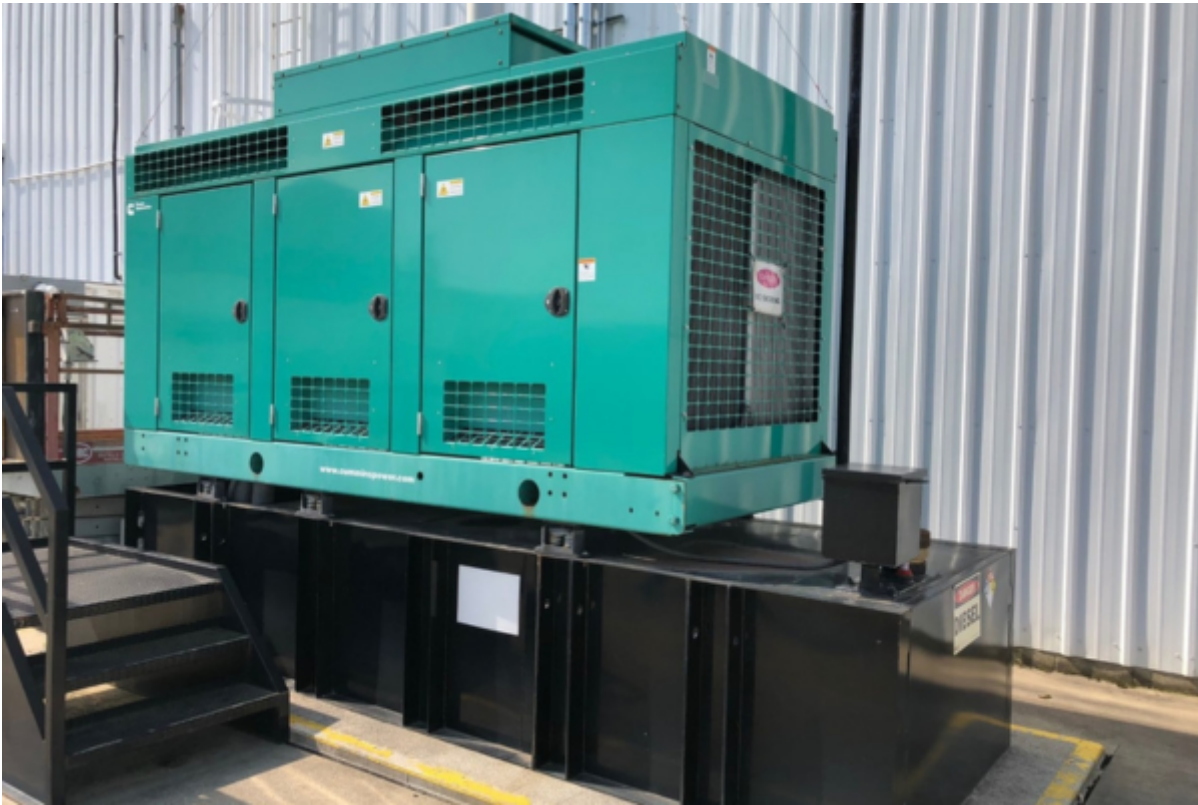
Industrial Power Generators
